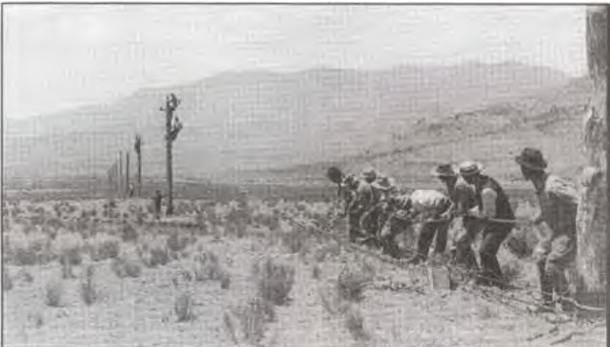
Construction crew stringing power lines for the first public power plant in Lincoln County. Collection of Donald Queen, Carrizozo, New Mexico.
